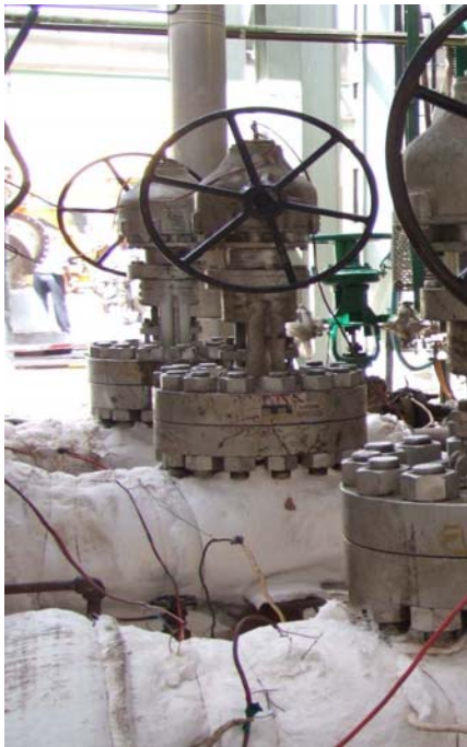
Photograph of Letdown station
