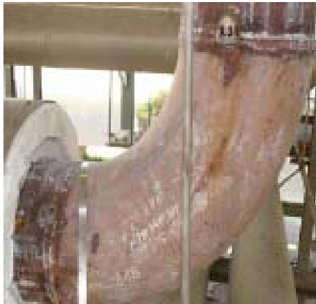
Replica location in Main Steam line
