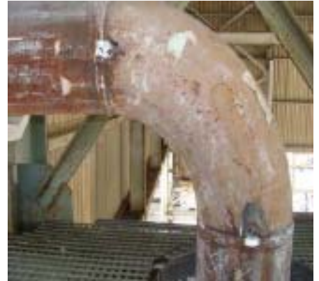
Replica location in main steam Near Co2 compressor floor
