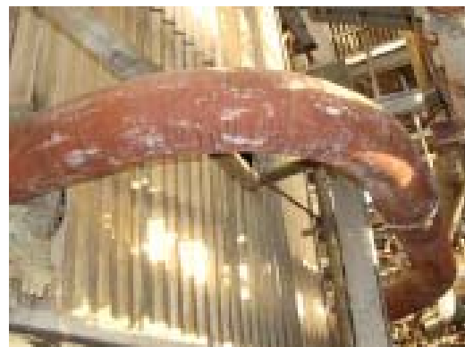
Main Steam line
