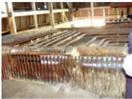
DPT on Top Front Header Stub joints
