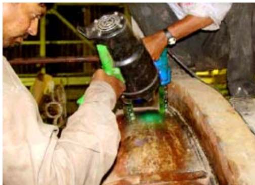
MPI in Steam Drum Dish End Circumferential seam
