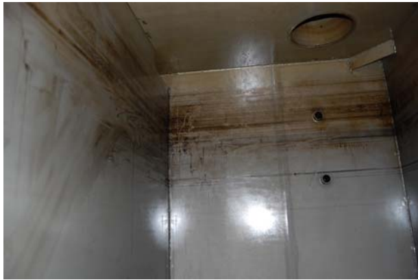
FIG 5, Deposits on side wall of LO Console
