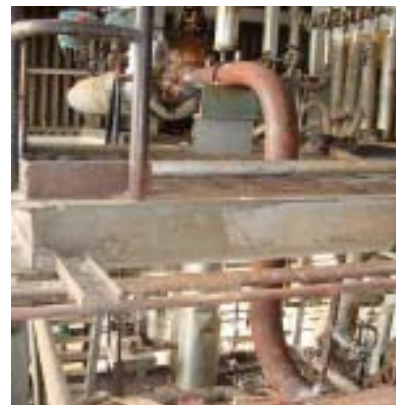
Feed water line
