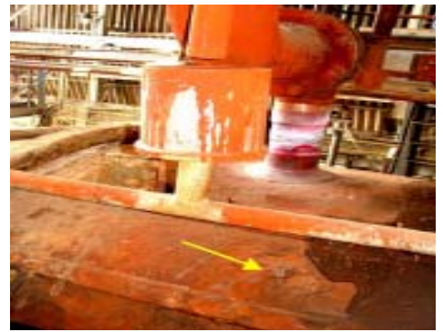
Corrosion spot on Steam Drum
