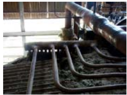
Top Rear Header & Riser Tubes
