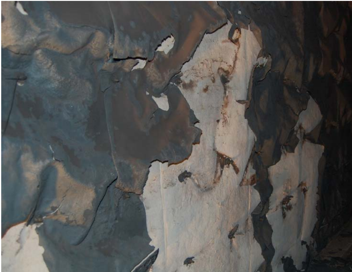
BEFORE: DAMAGED INCOLLOY 800-H LINING
