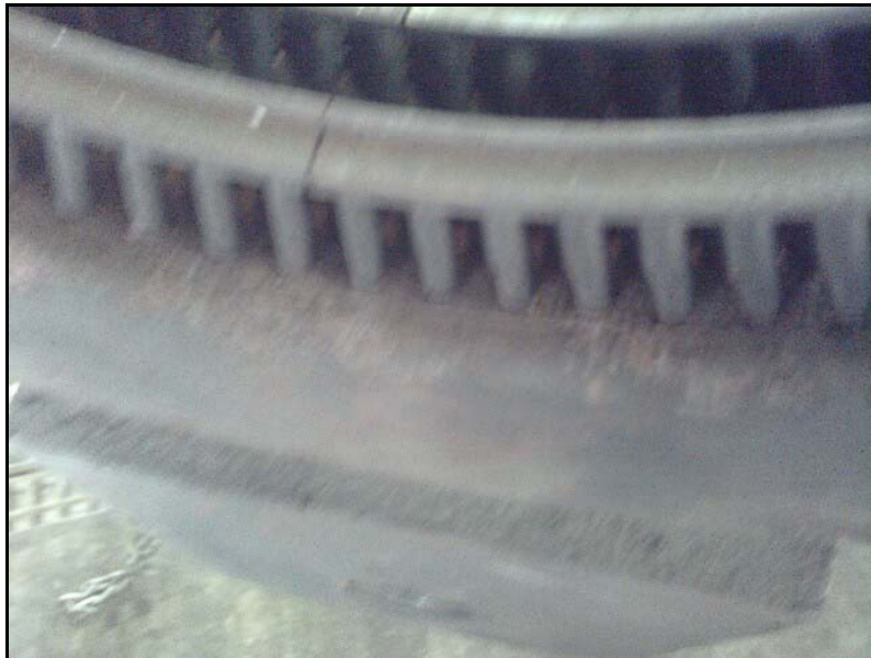
Figure -7: Pitting observed on GBC-2
