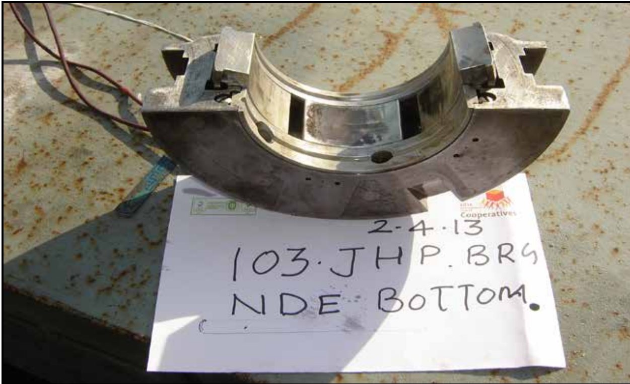
THICK BLACK DEPOSITS ON BEARING PADS OF 103-JHP
