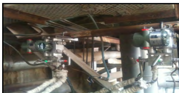
Anti surge flow indicating transmitters FR-1801
