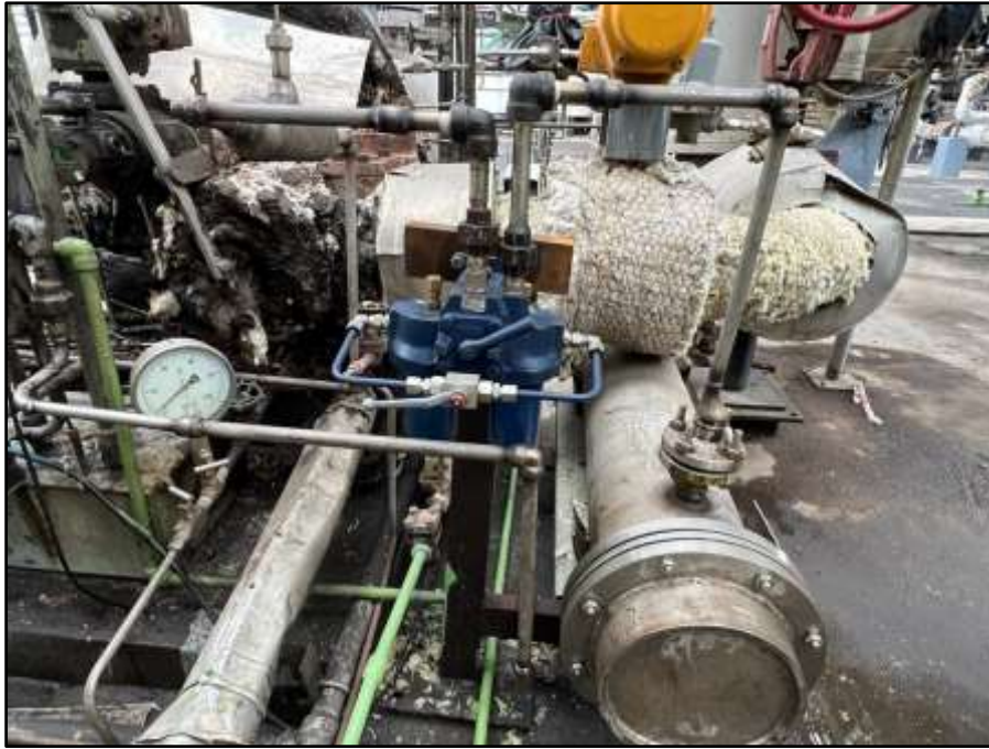
Lube oil Cooler with new Duplex Filter assembly installed in cooler outlet line
