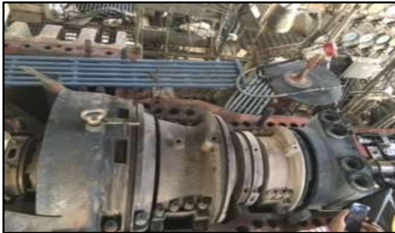
View of turbine After removal of Top casing cover
