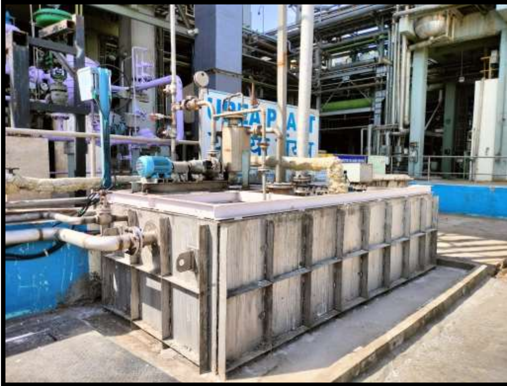
New underground ammoniacal water tank
