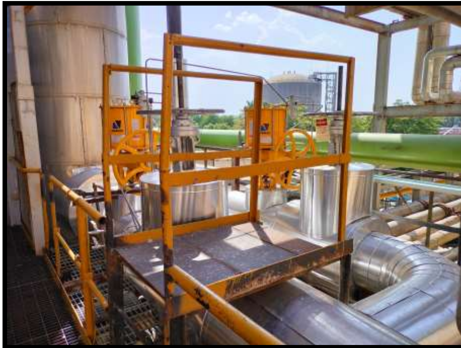
Split pressure control valves
