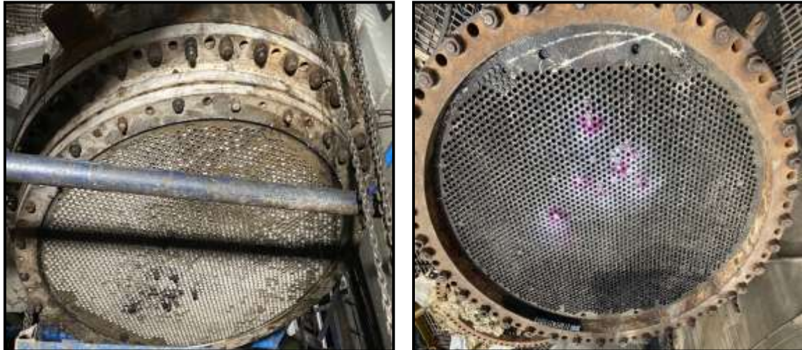
8 nos. leaky tubes plugged in 105-CB (Tube #51/14, #50/16, #49/24, #45/25, #44/30, #39/22, #39/26, #29/21. Rows marked from silo side
