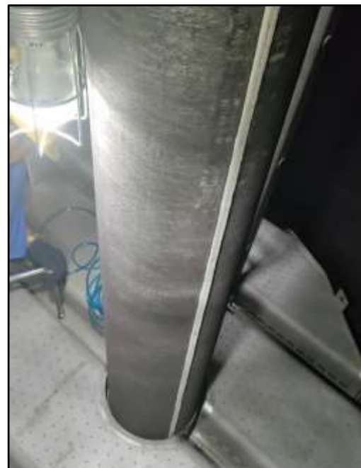
Downcomer line condition
