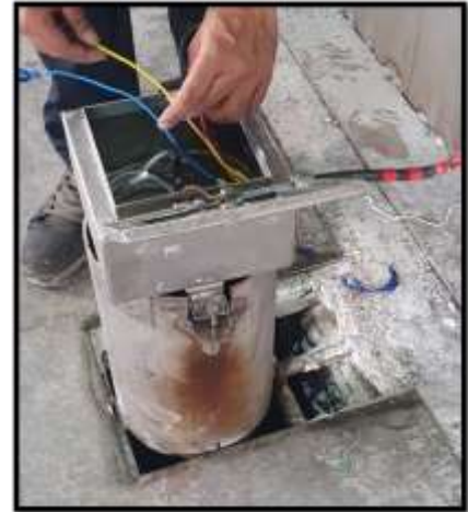
Nozzle and JB for level switch
