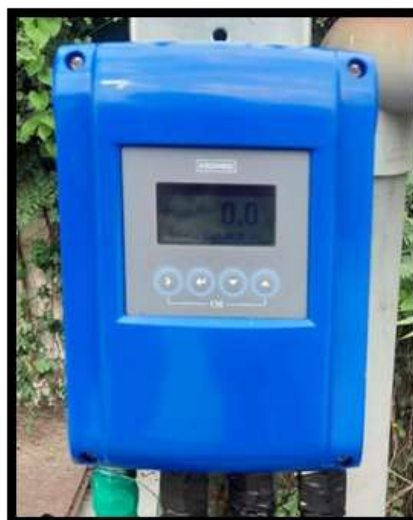
FI-6200 Transmitter / Flow indicator
