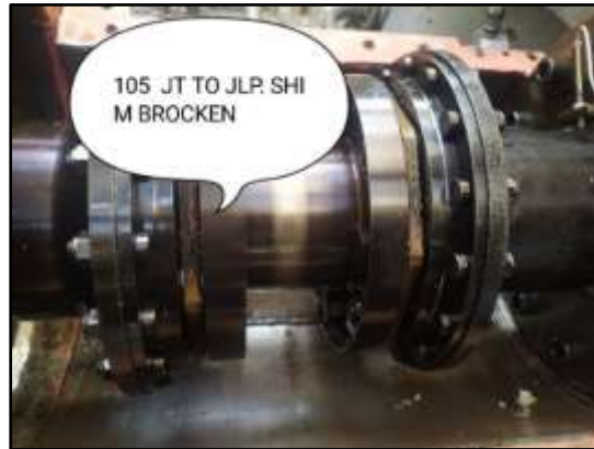
Damage of coupling Shims between Turbine to LP compressor.
