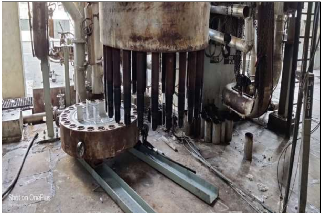
Bottom manhole cover removed and placed on Hillman roller
