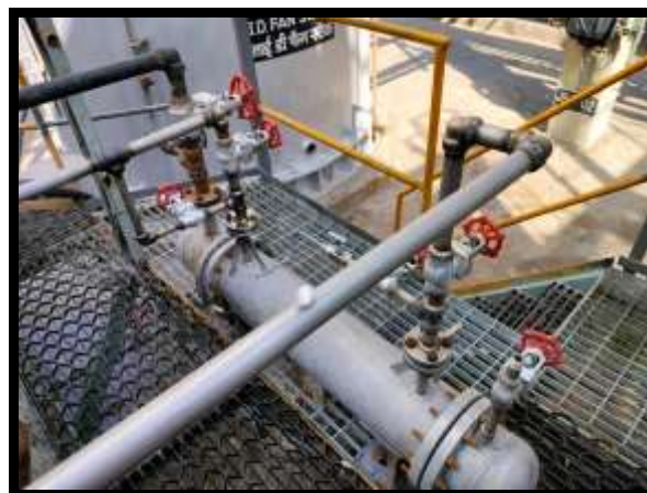
Additional lube oil cooler
