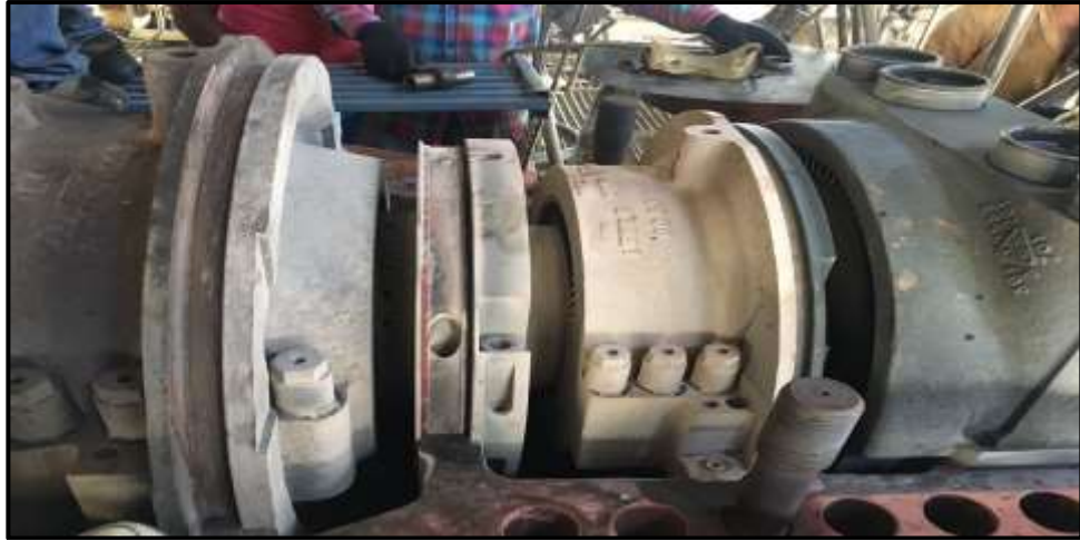
Scaling observed in above picture
