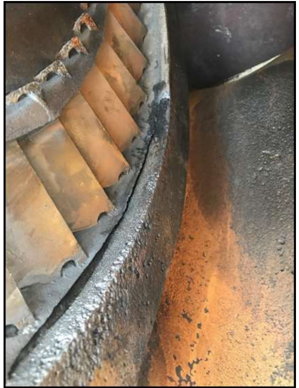
Pittings observed in stage
