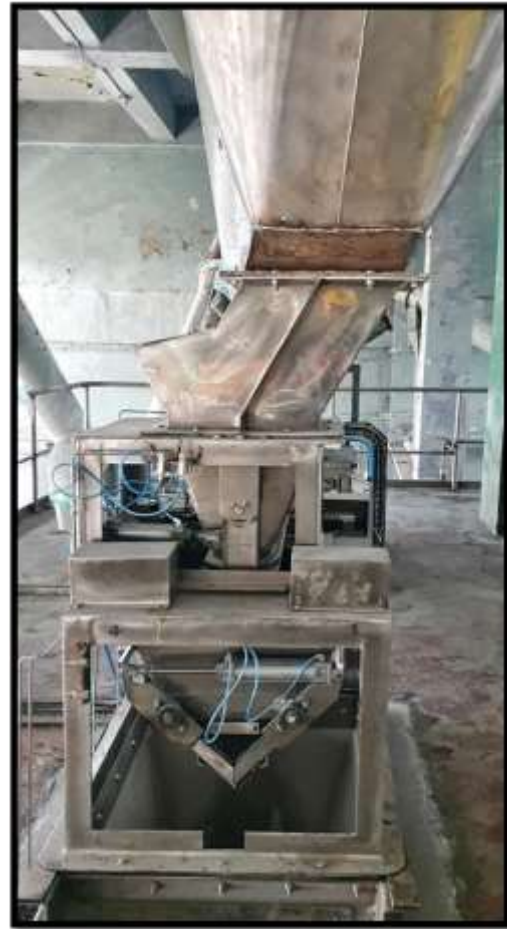
Bagging Machine Side view
