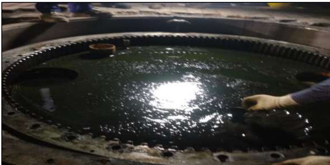
After removal of scrapper arm, condition of slewing bearing.
