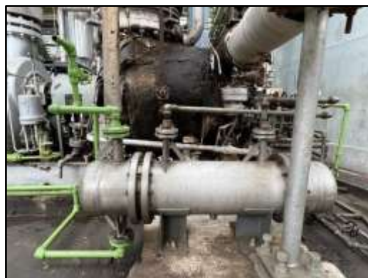
New lube oil Cooler of 104-JAT
