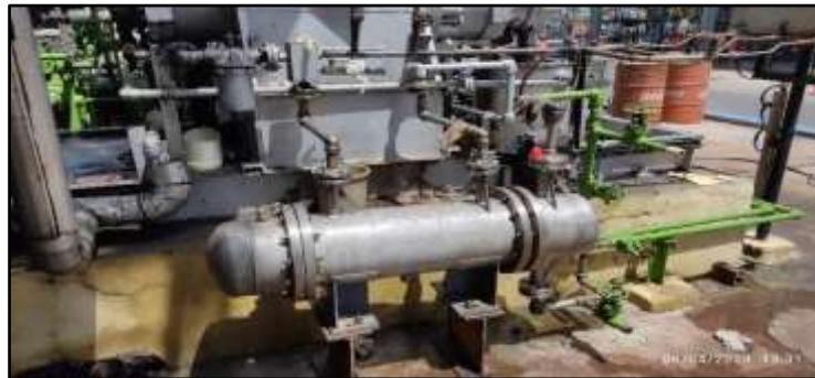
Replacement of damaged part of duct and Lube oil cooler of P-5111 is replaced
