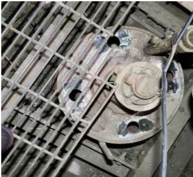
Arch burners damaged studs cut
