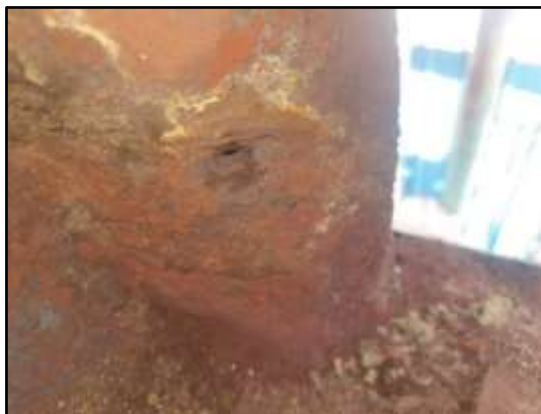
Pinhole at deaerator downcomer line
