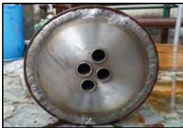
2 nos. of tube expanded at works of M/s Patel Air Temp and 2 nos. of tubes expanded in urea maintenance site
