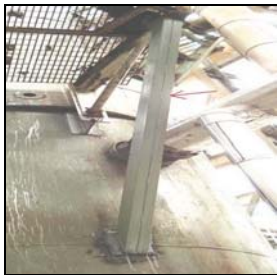
FICV-14 d/s Line support rectification
