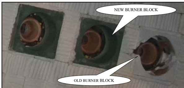
NEW BURNER BLOCKS
