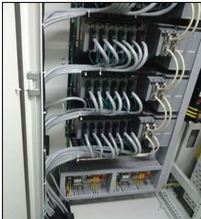
Prefab Cable connections in DCS System
