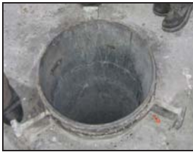
Extended portion of of drop out nozzle pipe (after removal of refractory)
