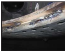
Gap was filled by welding. Plates were inserted and welded wherever gap was more.
