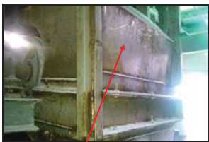
SS discharge hopper (from M-1403-2 to M-1419)
