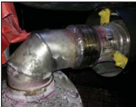
Expansion joint of quench line pipe
