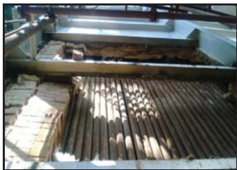
REFRACTORY REMOVED PANELS WITH DAMAGED BRICKS
