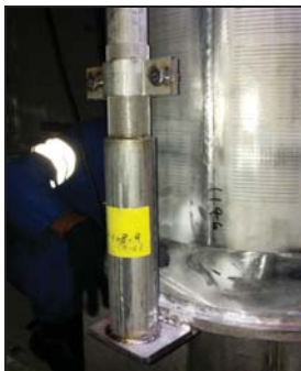
Bottom support of AT thermowell pipe
