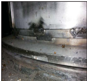
Gaps of 3-5 mm observed between support ring and collector bottom
