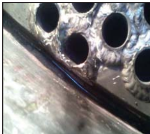
LEAK DETECTED AFTER HYDROTEST
