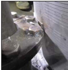
In 3 rd bed the flange of stuffing box was required to cut slightly as there was no gap. Also the slotted plate which was damaged at that area was covered by providing plate.
