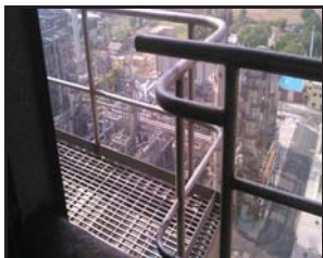
New SS 304 Platform -1
