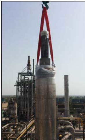
122- C shell side gas inlet portion and gas outlet pipe was covered at top
