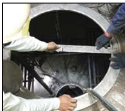
1 st , 2 nd and 3 rd bed ring centre was checked by using notch plate of required dimension
