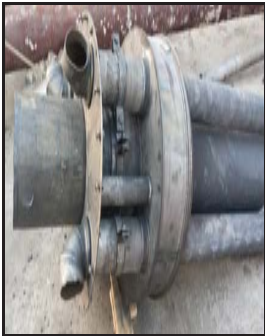
Removed Inner collector top piece
