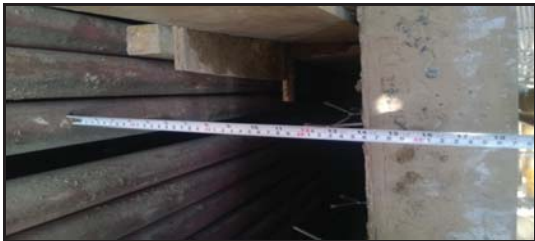
GAP SHOWN BETWEEN TUBES AND PANELS
