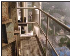
New SS 304 Platform -3
