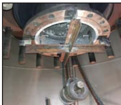
upto bottom manhole of convertor
