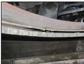
Gap between 1 st bed bottom dish end and cover
