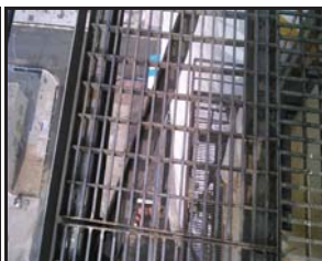
New SS 304 Platform -4
