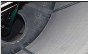
2 nd bed outer collector and bottom manhole
