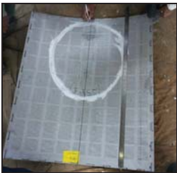
Marking done for panel on inspection hole. Marking for stitch welding was done on all panels
