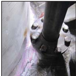
Stuffing box packing for thermocouples at 1 st , 2 nd and 3 rd bed was replaced
