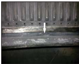
Cracks were observed in stitch weld between perforated plate of top outer collector bottom portion and the existing support ring
