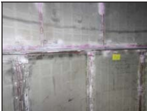
4 th bed bottom outer collectors after replacement of bottom outer collector and perforated plates of top portion
