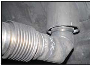
Expansion joint of quench line at 1 st bed
