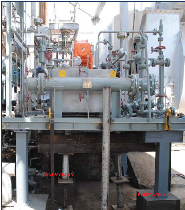
ERECTED LUBE OIL SYSTEM
