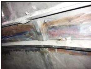
New support ring for protection screen which is below the existing support ring
