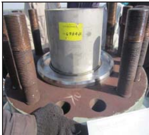
Special gasket & outlet insulation sleeve in position
