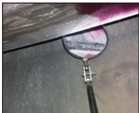
Cracks observed at back side portion
