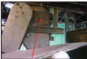
SS discharge hopper (from M-1421 to M-1419)
