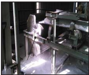
SS discharge hopper
