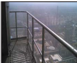
New SS 304 Platform -2
