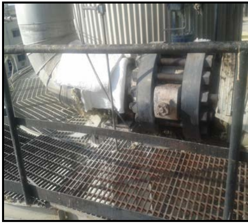
HIC-487 valve d/s flange weld joint leak location
