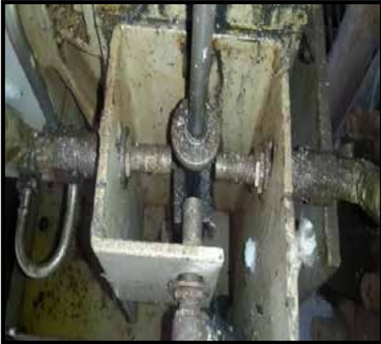
Proximity switches installed with Square shaped Target block
