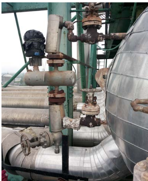
Old Level Transmitter Installation
