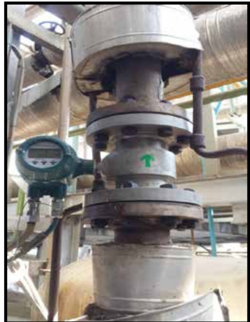
Magnetic flow meter FRCT-1421
