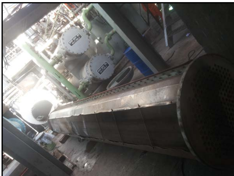
Broken studs on 129-JC
