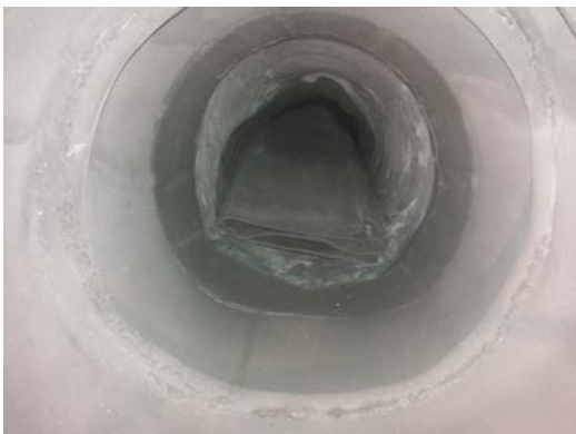
Damaged 103-D to 101-CA pipe Liner
