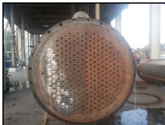
Total 28 nos. Tube is plugged in 130-JC
