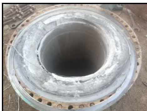
Damaged refractory at the top face
