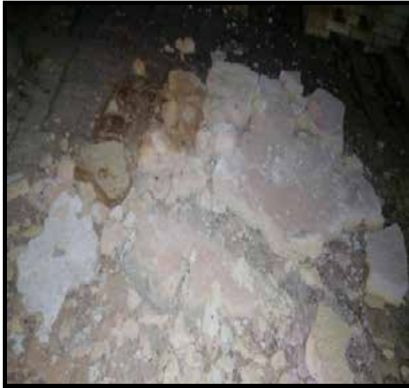
Refractory fallen on the floor.
