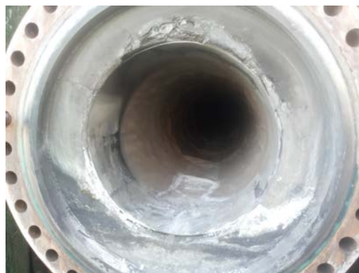
Damaged Refractory on seating area of Transfer Line End Plug
