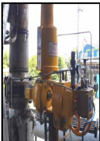
Control valve HICV-1406
