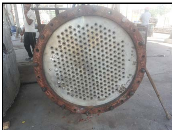
2 nos. Tubes Plugged in 129-JC
