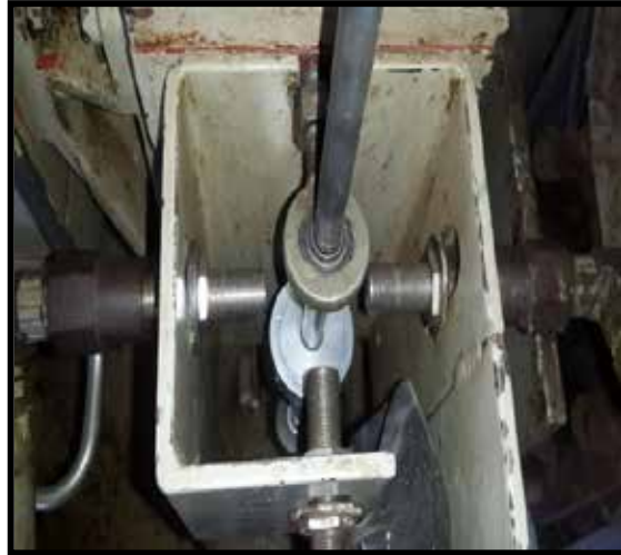
Proximity switches installed with Round shaped Target block
