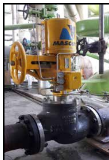
Control valve HICV-1204
