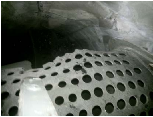
Damaged Distributor of 101-CB
