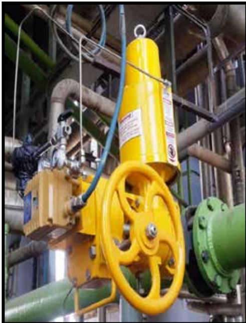
Control valve TICV-1226
