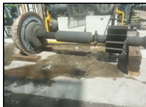
Existing 103-D Burner Assembly before Modification
