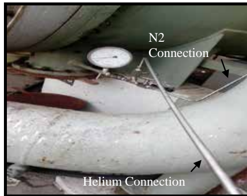
Connections for Nitrogen & Helium cylinders
