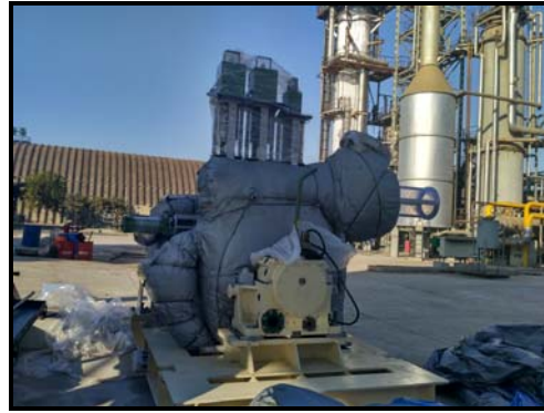
Front view of New Turbine
