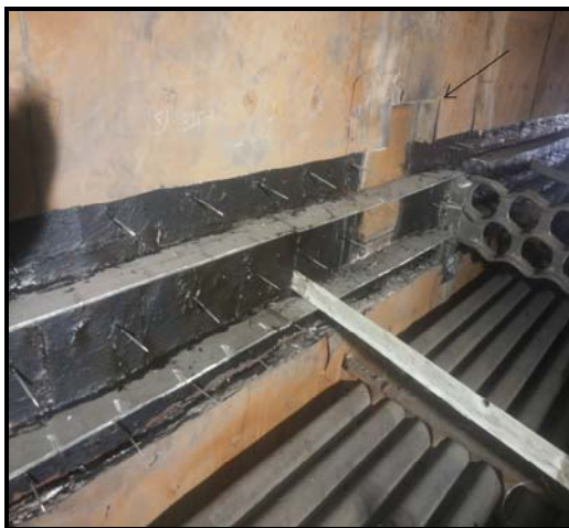
Retainer plate and studs provided on wall for insulation. Manhole above HT Coil is closed
