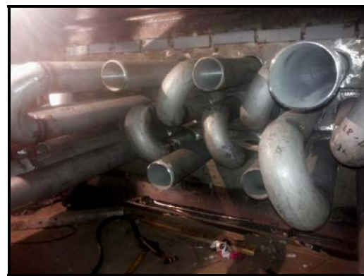
Header end of coil after insertion of coils
