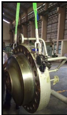
Discharge head cover removed from barrel
