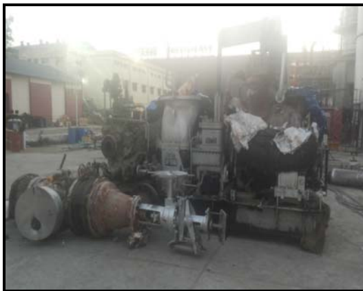
103-JAT and 103-JBT removed and kept on Ground floor
