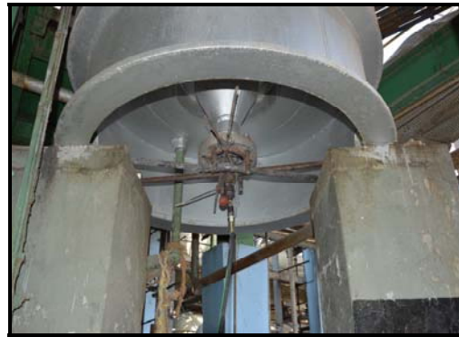
Burner provided at bottom of 101-CA/B
