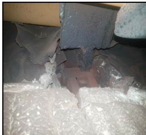
Damaged 3 rd ITS support
