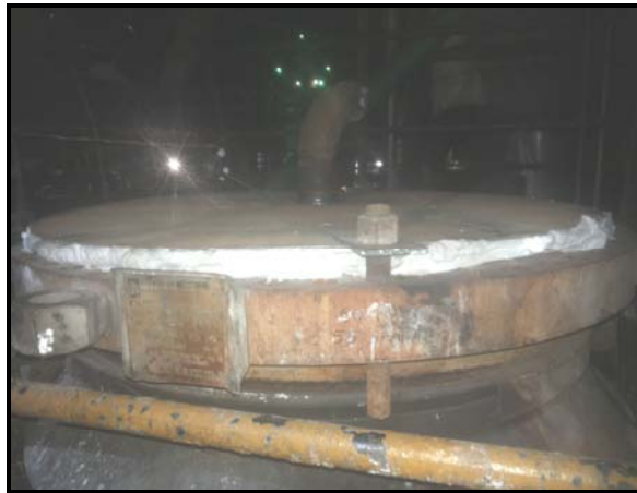
101-C covered with plate & exhaust provided
