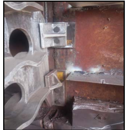
Supports of ITS
