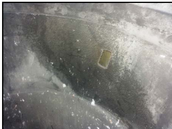
Shell liner removed from 101-C
