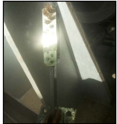
Earthing brush found completely worn out
