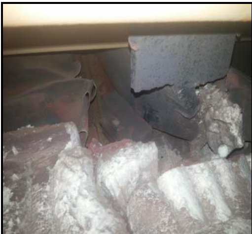
Damaged 2 nd ITS support
