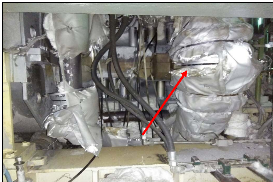
Flange marked in red color leaked during startup
