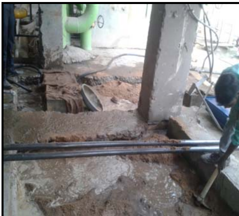
Pedestals of HPCOS & HP Oil Cooler
