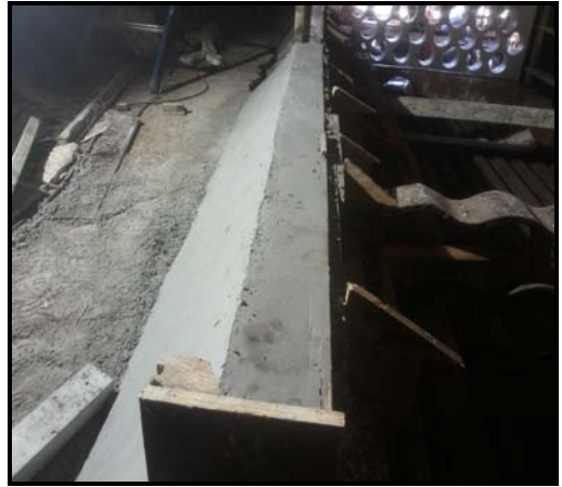
Refractory provided on wall 6
