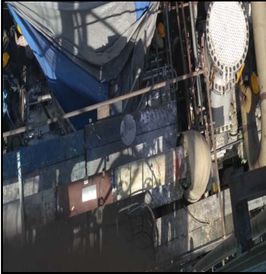
Flow nozzle in Steam inlet Line
