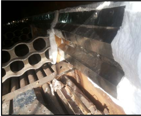
Incoloy sheet provided on wall
