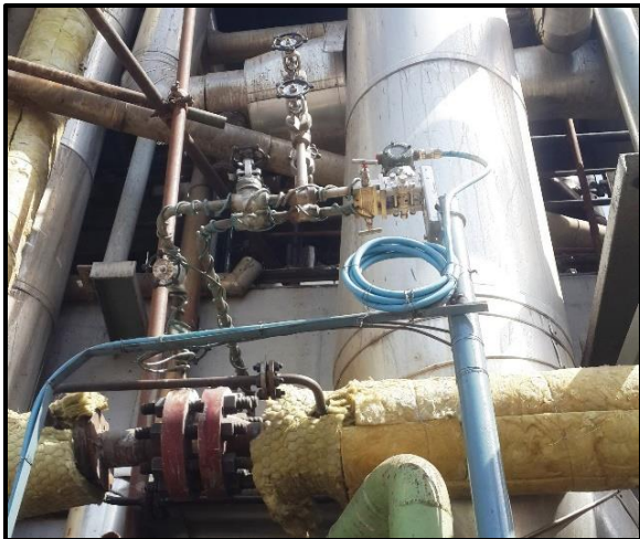
Flow element & DPT for FI-1206
