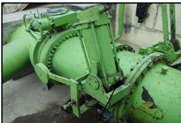
Old Check Valve
