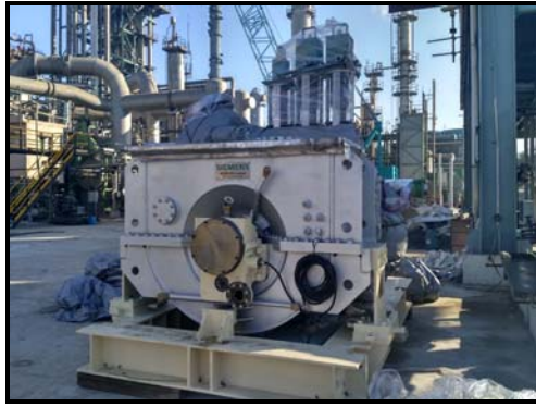
Rear view of New Turbine
