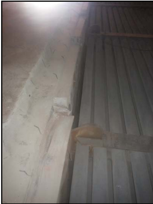
Existing refractory of HT to LT section of approx. width 250 mm was removed
