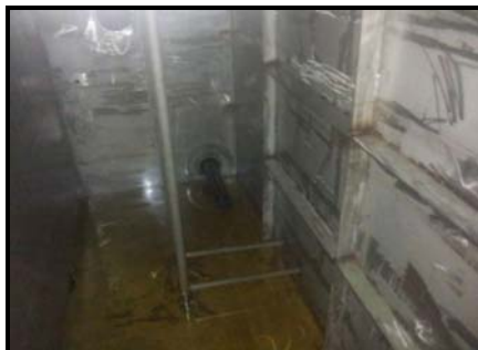
Inside view of LO Console
