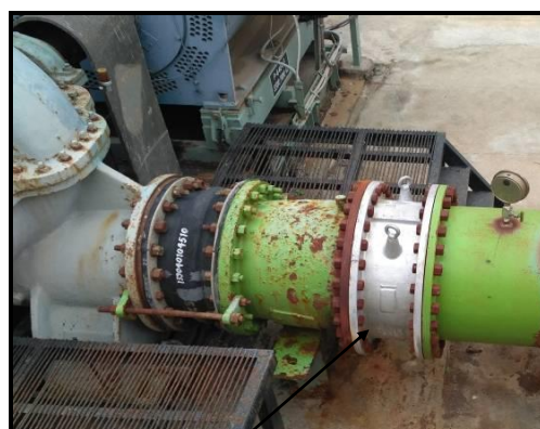
New Check Valve
