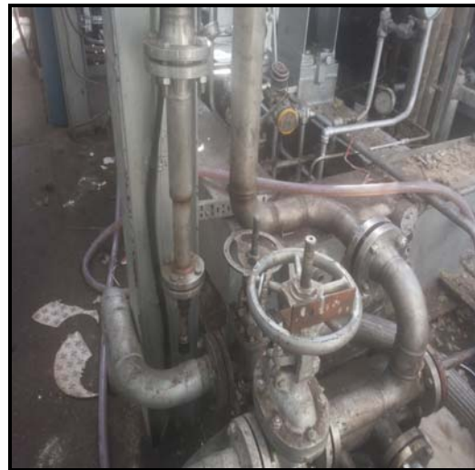
For flushing LO inlet header 101-J GO and LO lines bypassed
