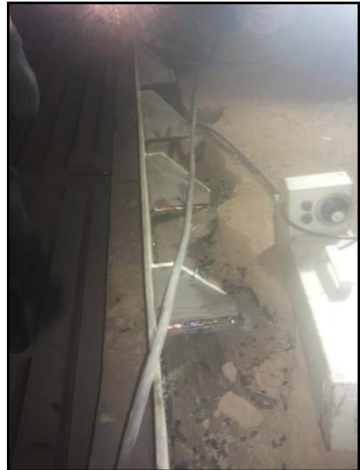
ITS Guides mounting plate with stiffener welded on HT to LT section wall
