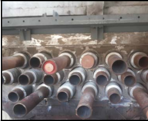
Outlet header end after positioning of coil
