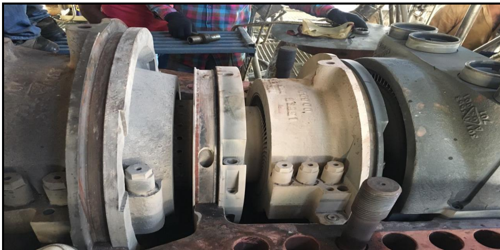
Scaling observed in above picture
