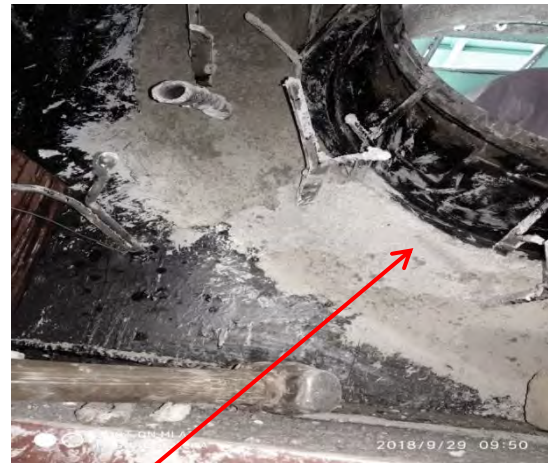
Insulyte-11 in port of burner block to match the level
