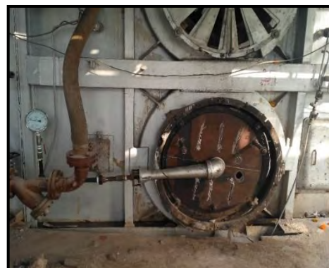
Temporary portable burner ( primary reformer tunnel burner )
