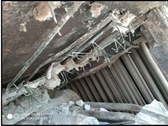
Top roof – 25% of top roof area was provided with castable supported with welded SS rods and hangers
