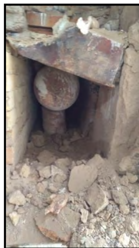
Retainer plate and refractory at north end of Coil B header was in damaged condition
