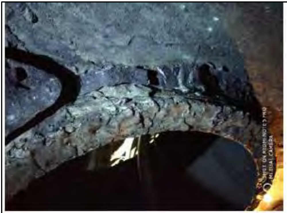
Putty applied on the circumferential weld joint of manhole nozzle with shell from inside was found detached
