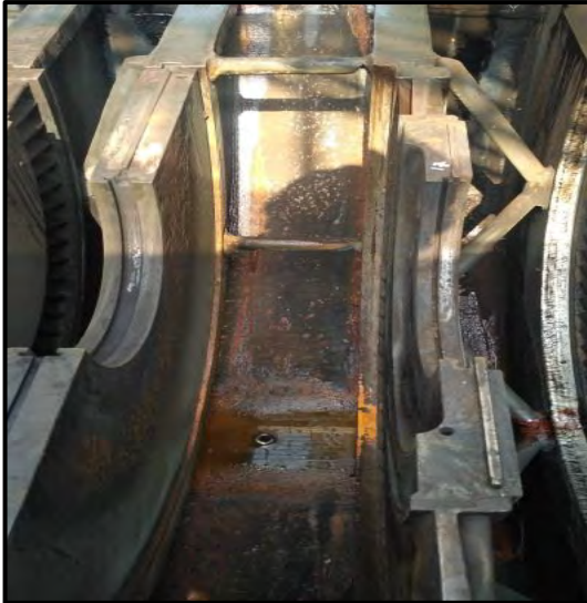
Eroded Reinforcement Rod
