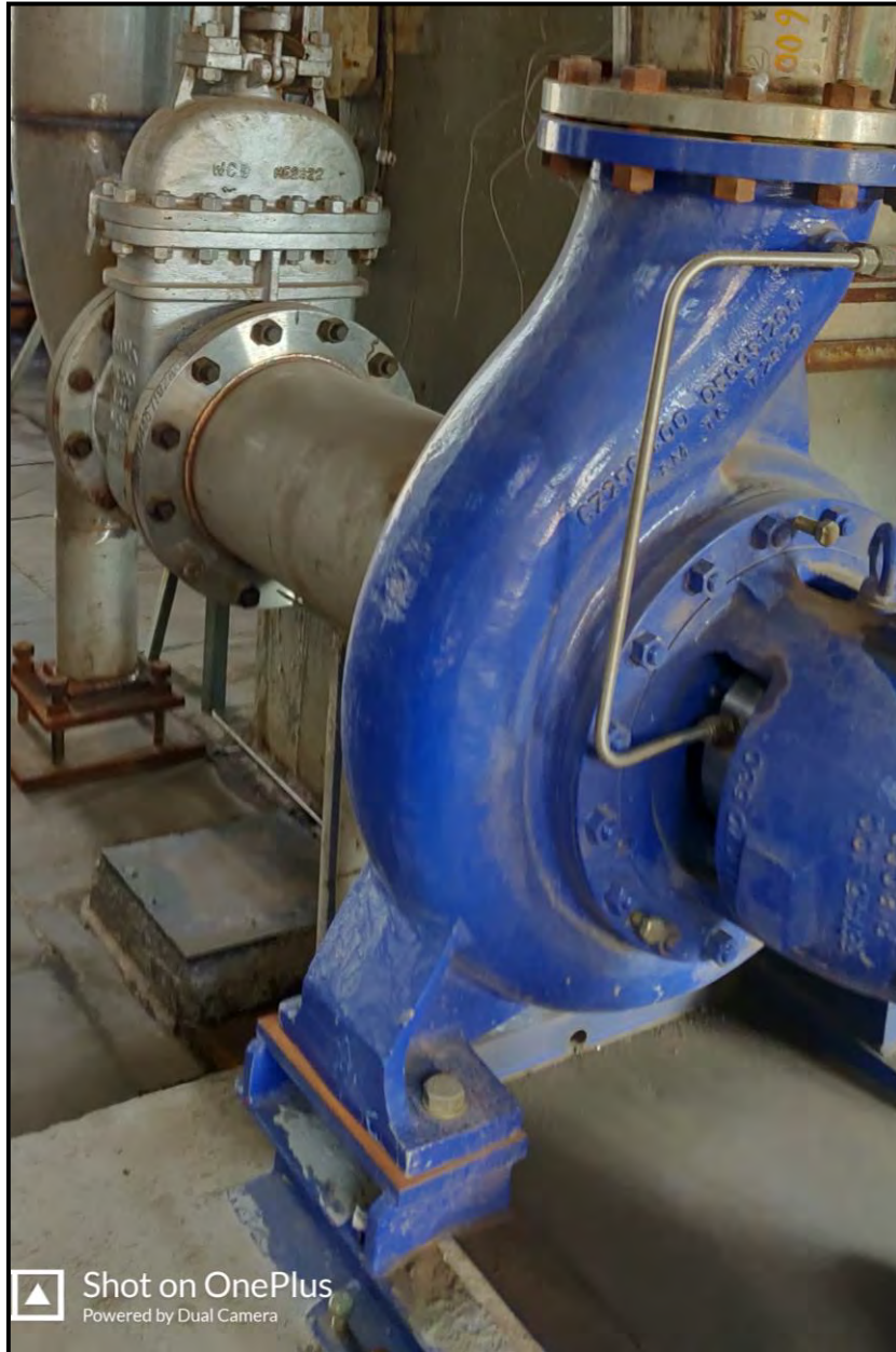
NEW PUMP P-1202-B, SUCTION LINE, DISCHARGE LINE & BASE FRAME
