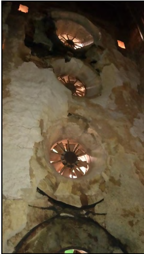
Damaged Refractory of front wall
