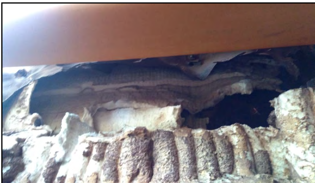
Damaged area of insulation below MFC coil
