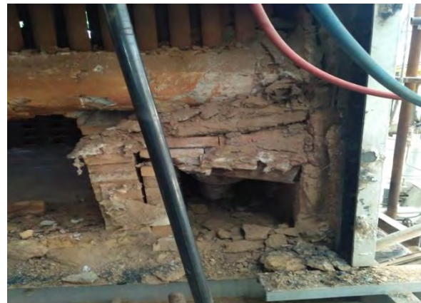
Damaged tunnel brick ( birdge wall ) with back wall
