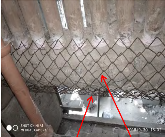
Coil C Header – new MS Mesh & Old welded anchors
