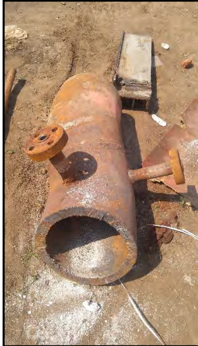
Removed outlet spool piece
