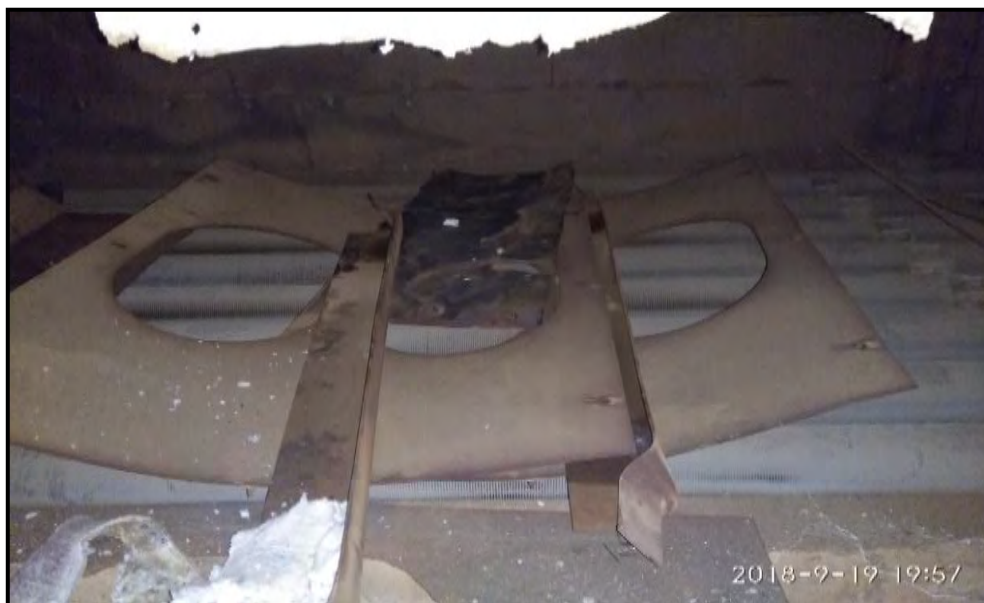
Baffle plates of transition zone
