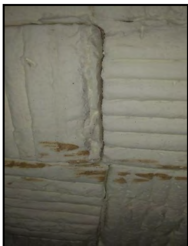
Gap observed between blocks
