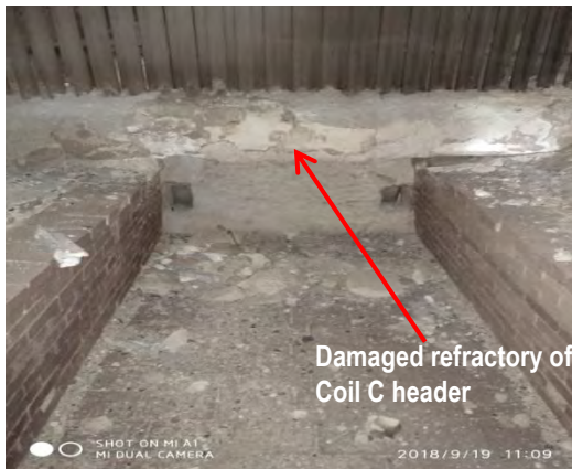
Damaged refractory of coil C header
