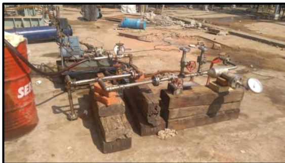
LO lines of Additional AOP was flushed
