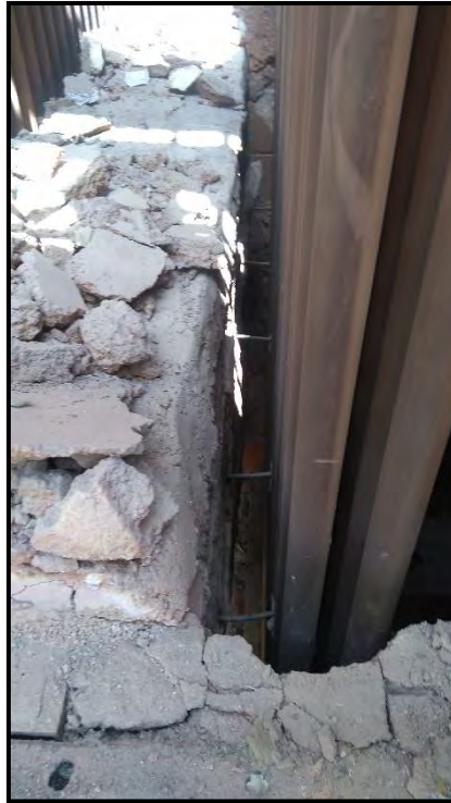
Damaged refractory of Wall #9
