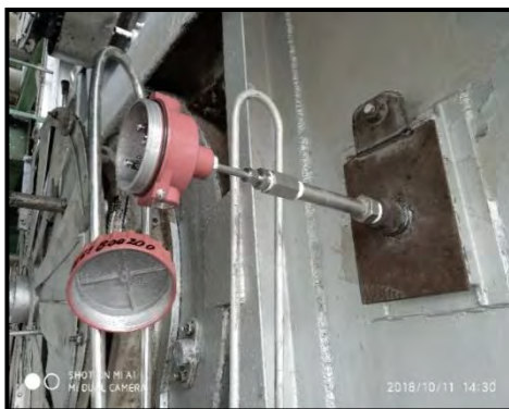
Temporary Thermocouple fixed in peep hole
