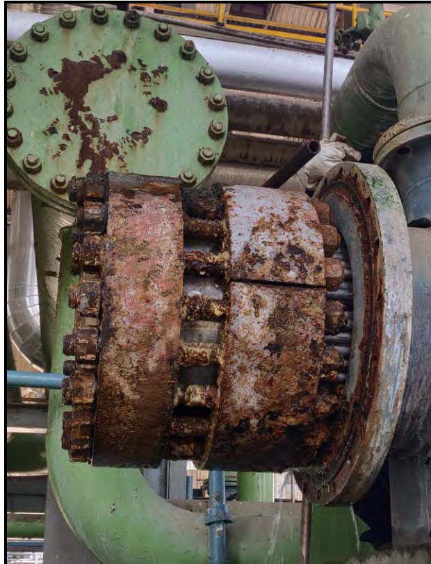
FLOATING HEAD COVER JOINT LEAK
