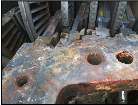
Eroded Moisture Rings
