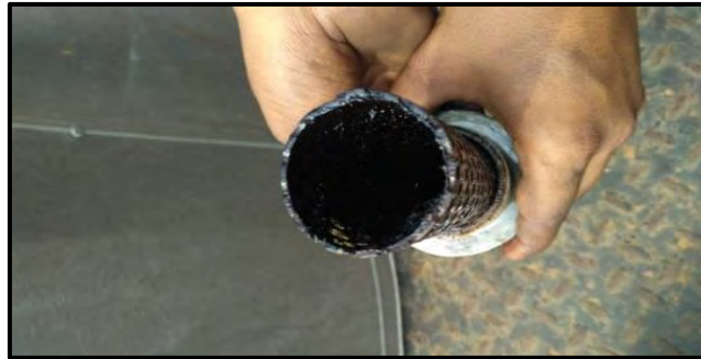
Choked strainer of 105-J seal oil line
