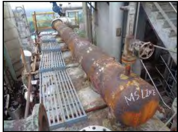
RLA OF MAIN STEAM OUTLET LINE
