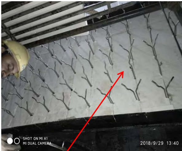
From top of 5 th burner – New anchor with ceramic board
