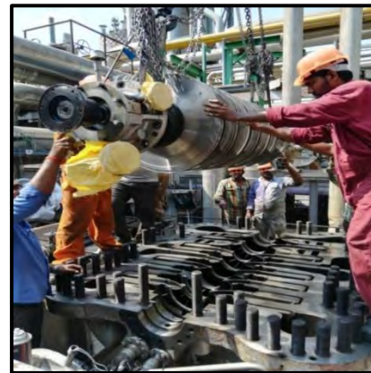
Placement of Rotor
