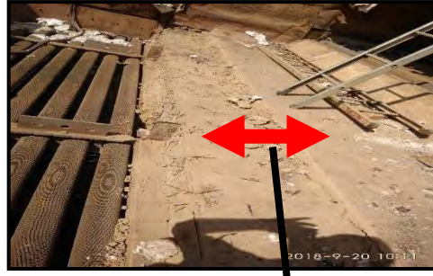
Broken the refractory upto 600mm on bridge plate
