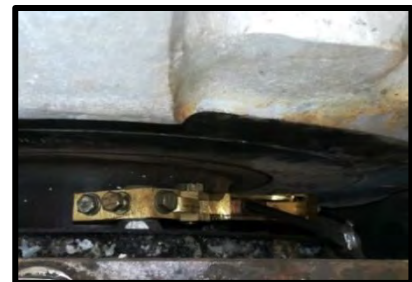
New additional Carbon Earthing brush
