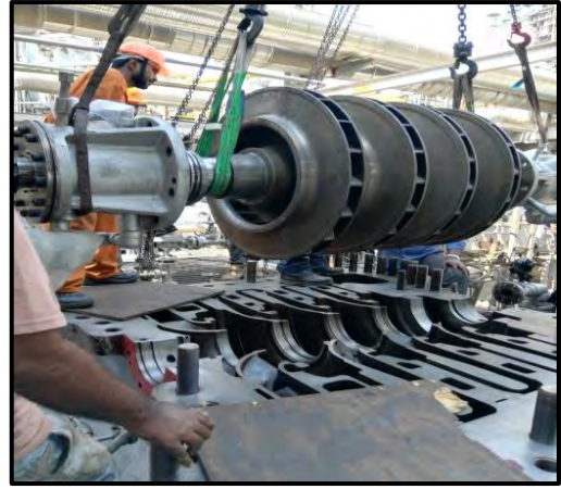
Placement of Rotor
