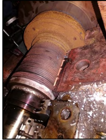
Balancing drum & seal found corroded & eroded
