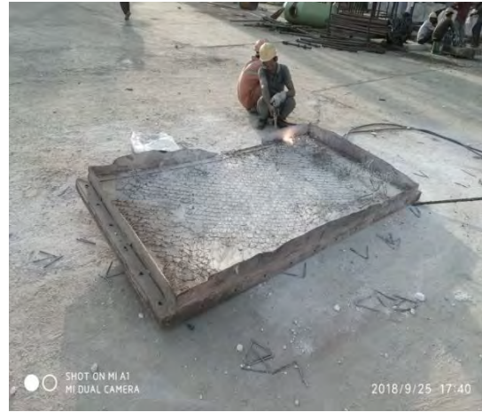
Damaged side plate cutting from panel
