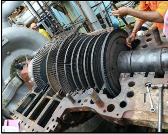
Initial Clearance measured before rotor removal
