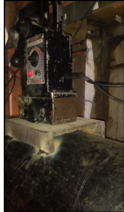
Online drilling for thermowell
