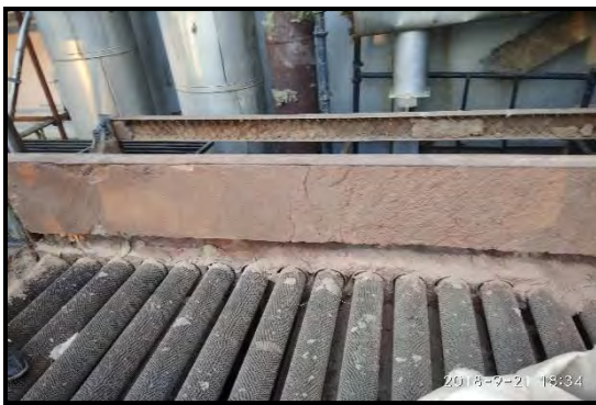
Refractory broken at 500 mm of BFW ETS
